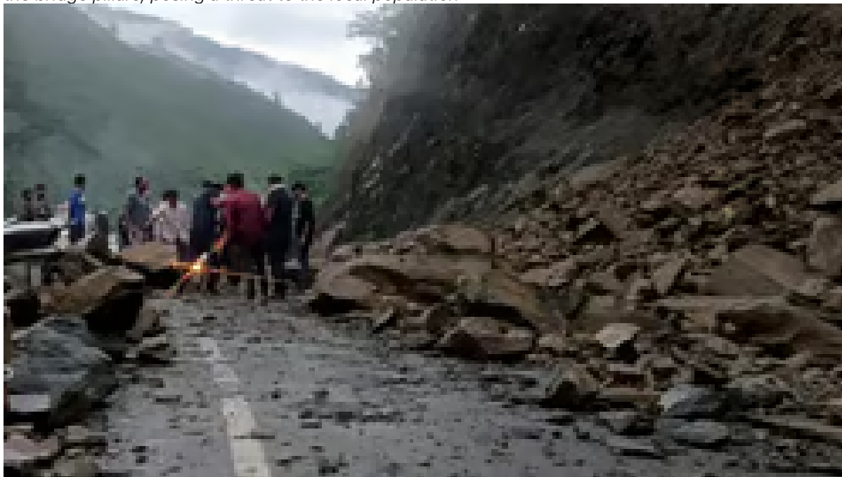
Debris being cleared from a highway following a landslide, in Uttarakhand's Chamoli district (Photo | PTI)
